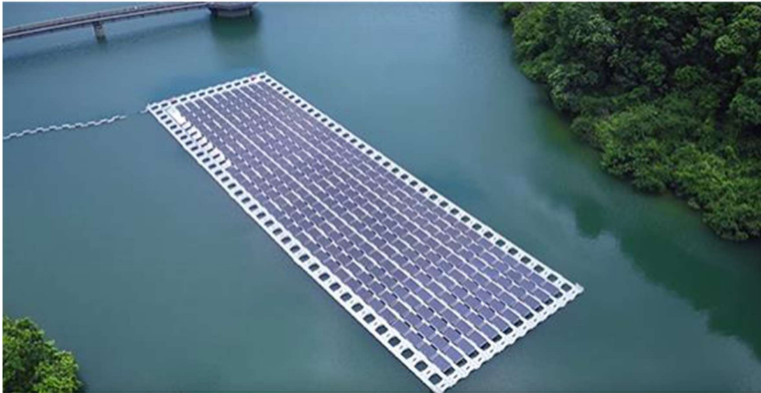
Solar panels installed on the water surface of a reservoir
