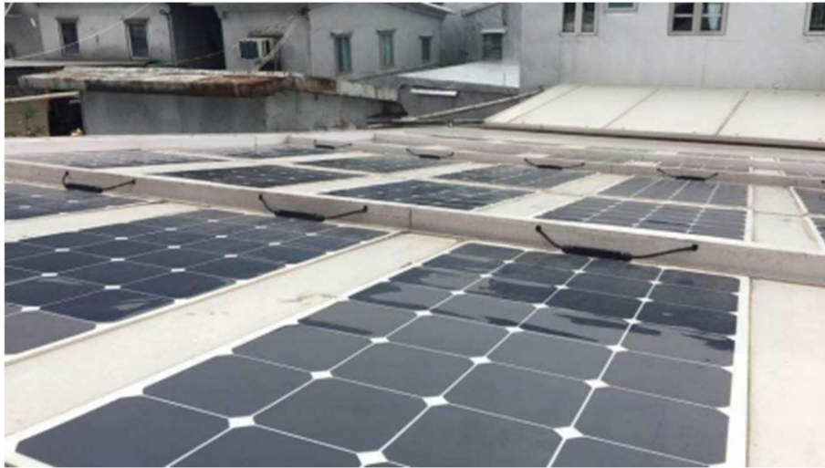
Solar panels installed on the rooftop of a village house in New Territories
